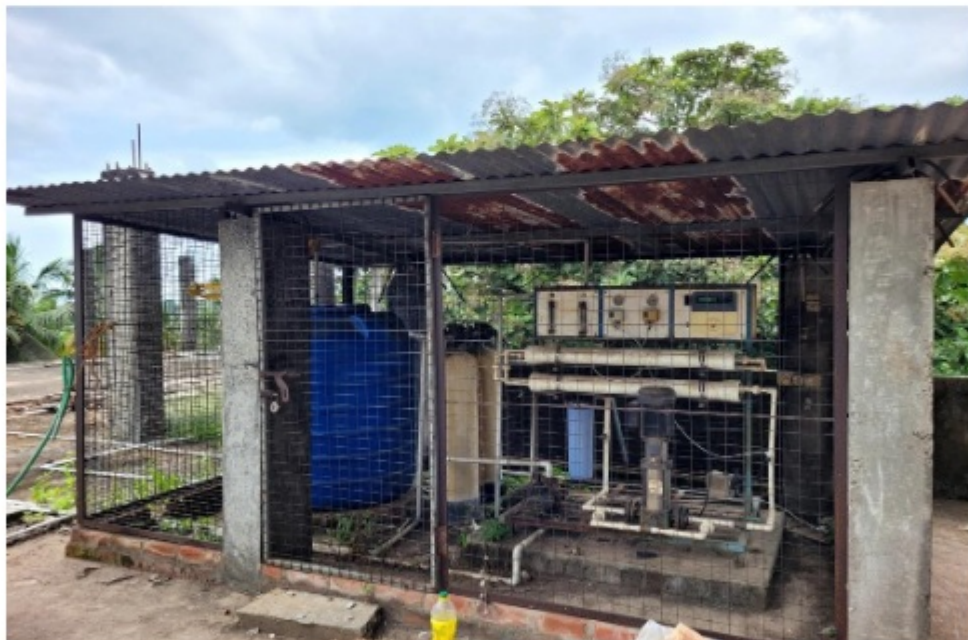
[Drinking Water Filtration Unit]
