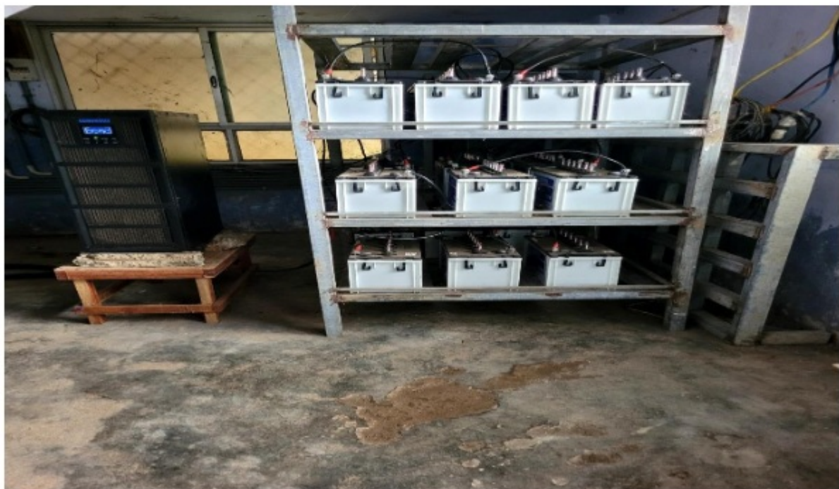
[UPS & Electrical Room]
